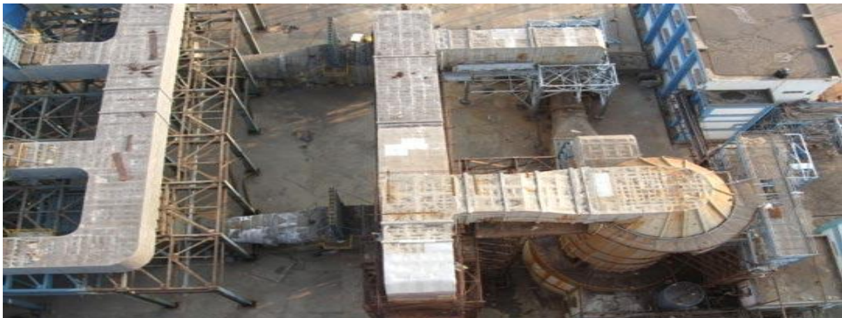
(India's first Wet limestone FGD system on coal fired power plant with production of saleable Gypsum for 2 x 600 MW Udupi Thermal Power Station, Karnataka, India. installed by Ducon)
